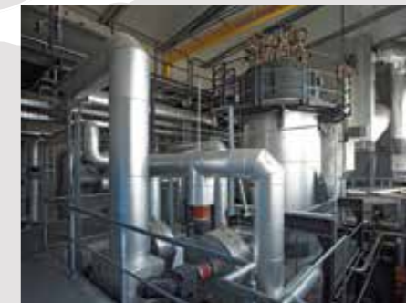
in-house biomass power plant
